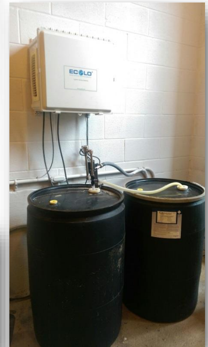
Drums with mixing dilution station
